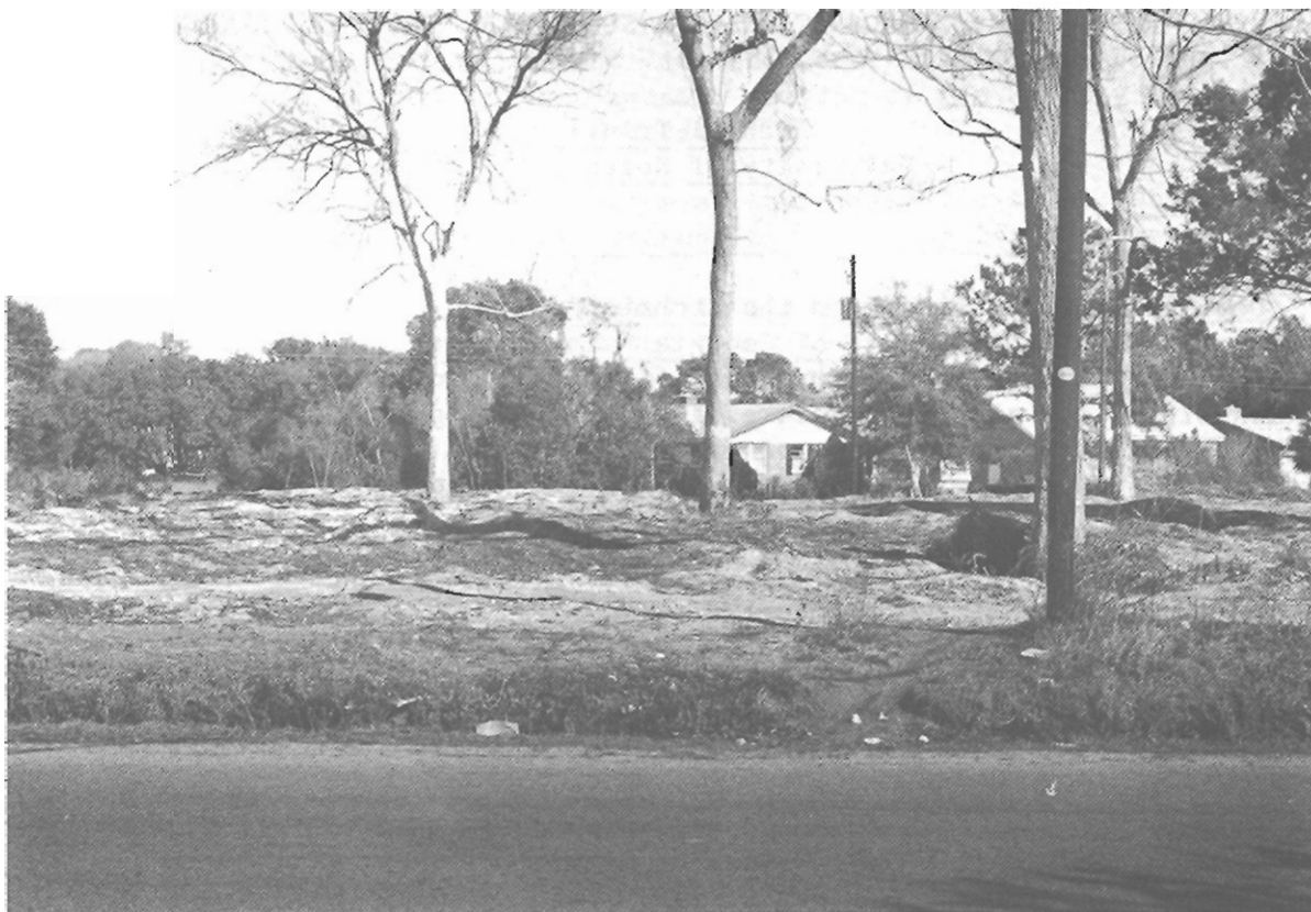
Figure 1. View of Lighthouse Point after being bulldozed. Looking toward the marsh (north).
